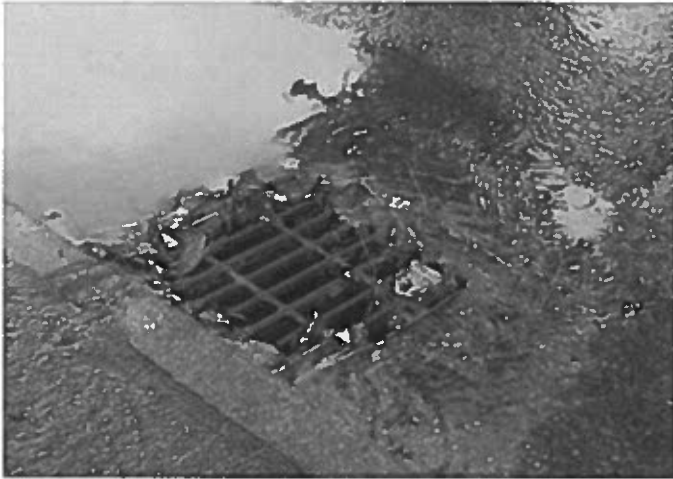
Storm drains carry rainwater directly to rivers and streams.
